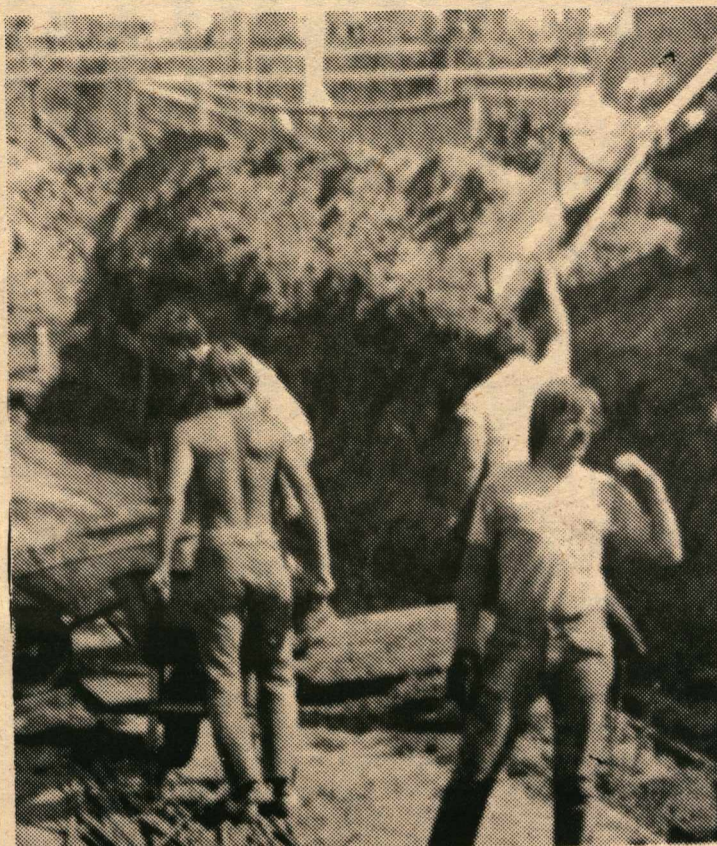
GMS workers pour footings for the combination church-parsonage building in Fort Smith, Northwest Territories, Canada. The group spent three weeks in upper Canada, working on the GMS project. This summer they plan to travel to Guatemala; applications for this GMS project will be presented in the General Missionary Society chapel in November.
